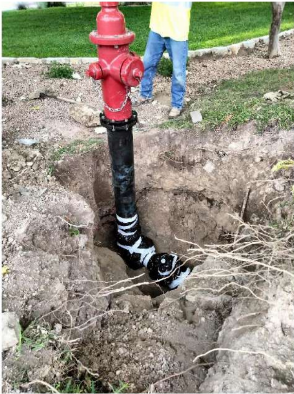
2024.04.16, Poly-wrapped Hydrant Piping
